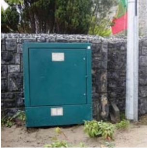
District Regulating Installation (DRI)
