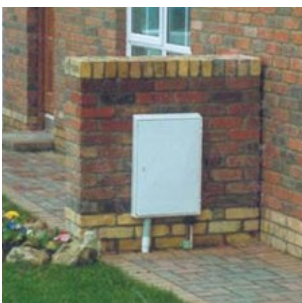
Domestic meter box
