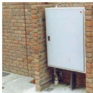
Six meter cabinet
